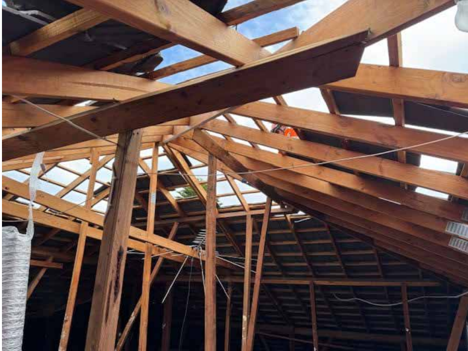
Roof damage to home - weather event 24 August 2025
