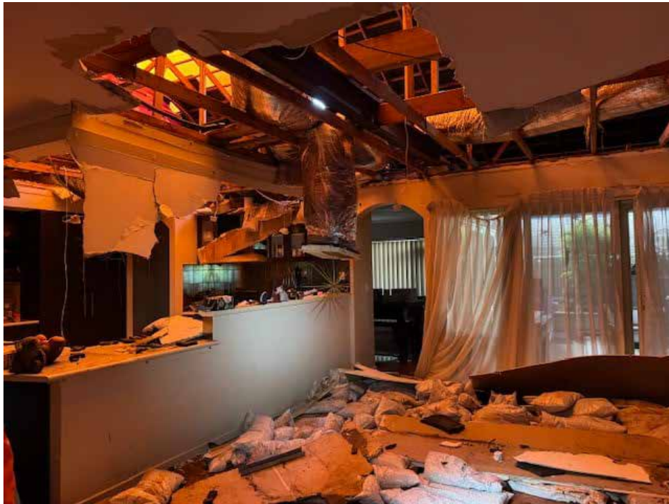
Internal damage to home - weather event 24 August 2025.
