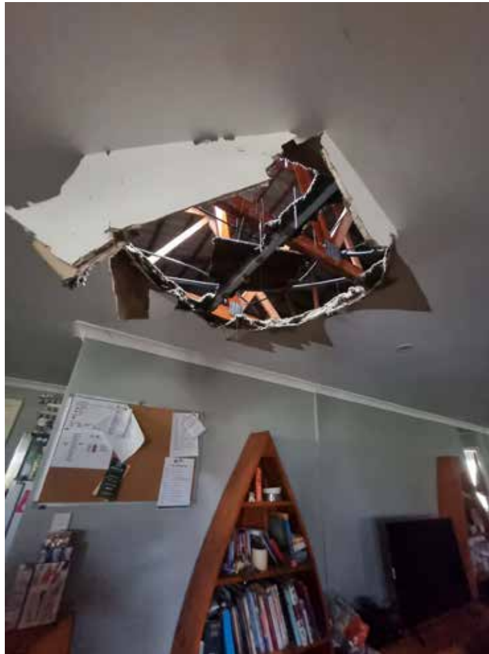
Example of Property Damage Encountered
