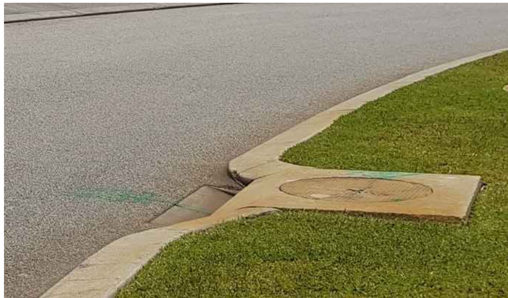
SIDE ENTRY PIT
