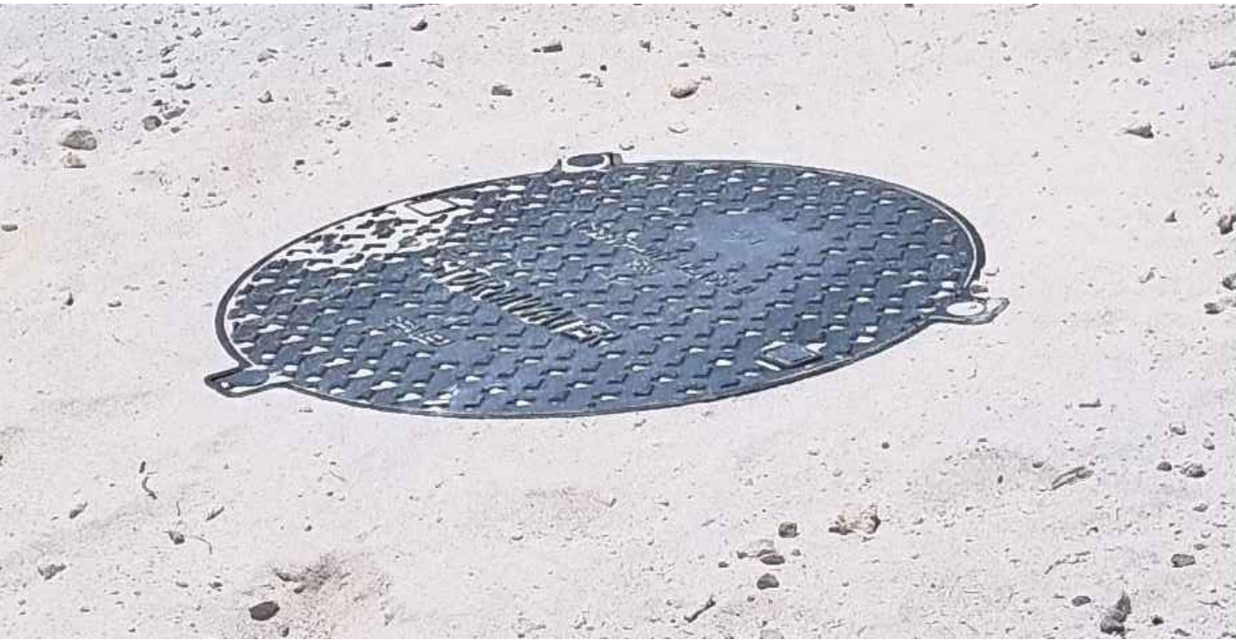
SOAKWELL WITH EXPOSED RAISED LID
