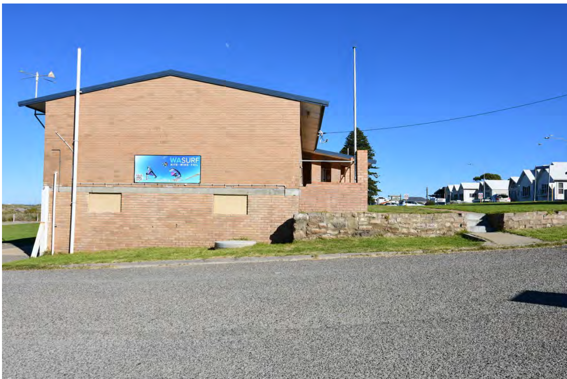
Photograph 4 The east elevation with structural repairs on the south east corner. Griffiths Architects, May 2026
