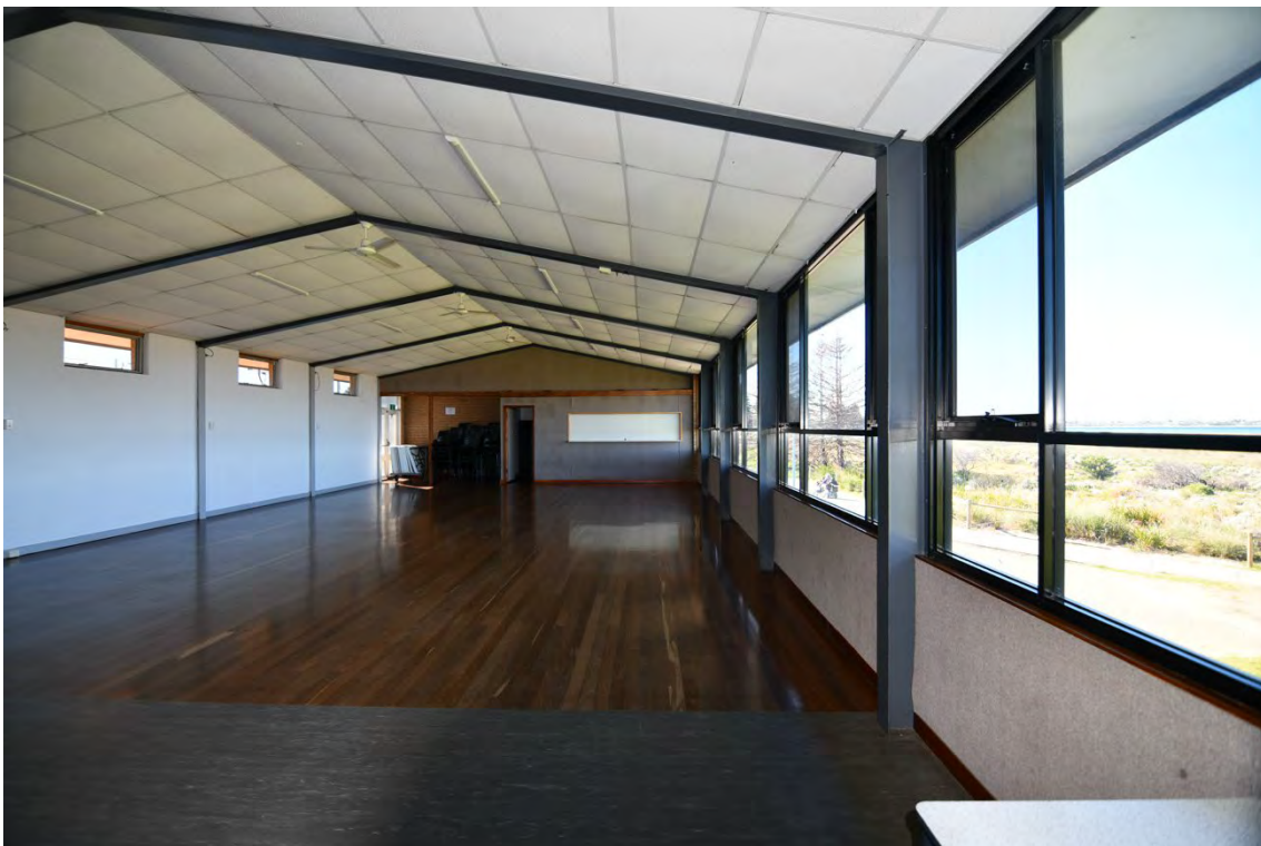
Photograph 13 Internal view of clubroom looking east showing portal frames and replacement windows, timber floors and mineral fibre ceilings. The bar was a later addition. Griffiths Architects, May 2026.
