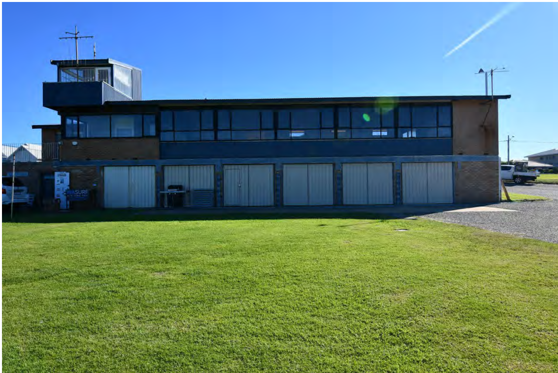
Photograph 3 South elevation with the later addition to the left. The brick piers have been reinforced and the lintel spans reinforced. Griffiths Architects, May 2026
