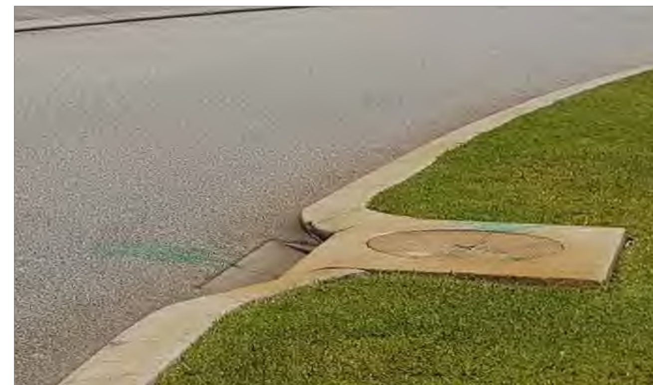
SIDE ENTRY PIT
