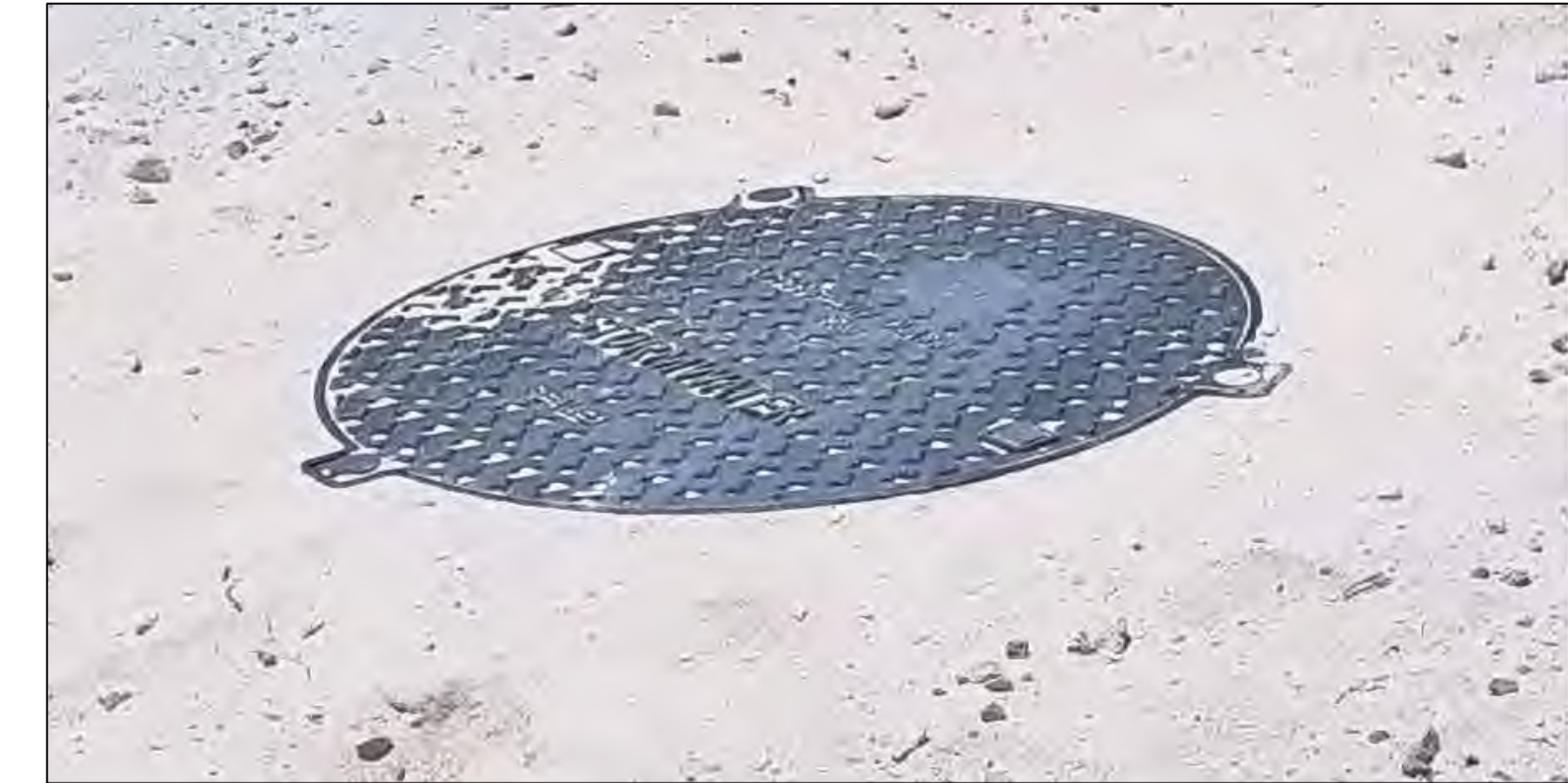
SOAKWELL WITH EXPOSED RAISED LID
