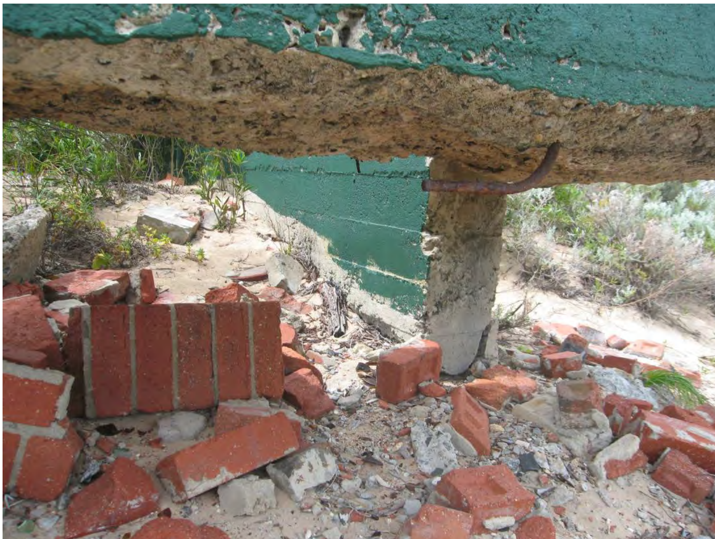
Figure 104: Gun Emplacement - underside of the concrete structure
