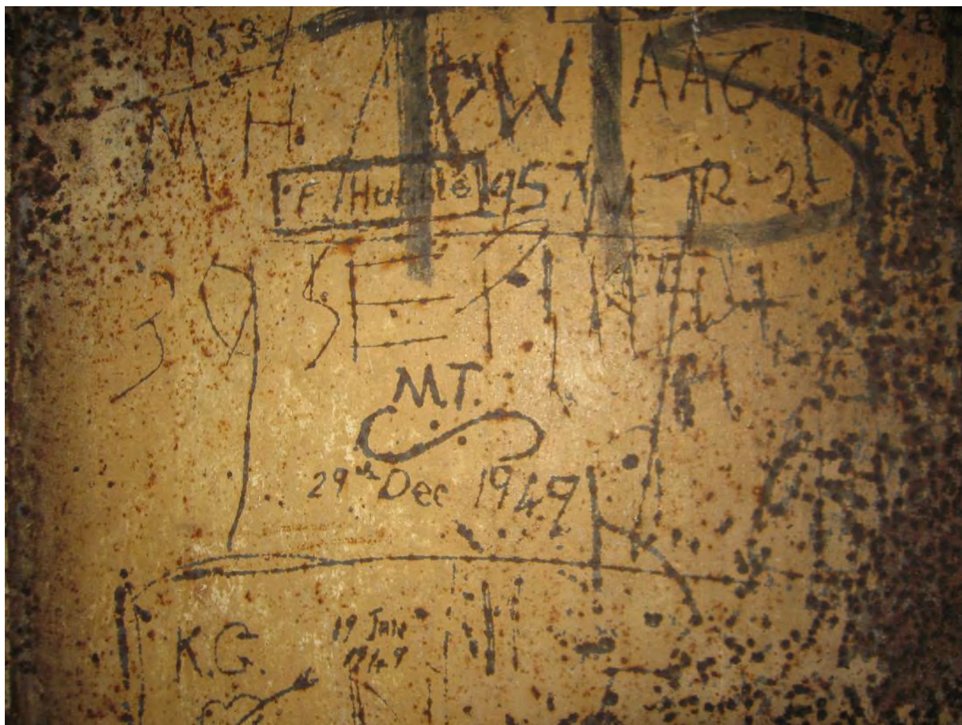
Figure 95: Operations Bunker – Graffiti scratched into entrance doors
